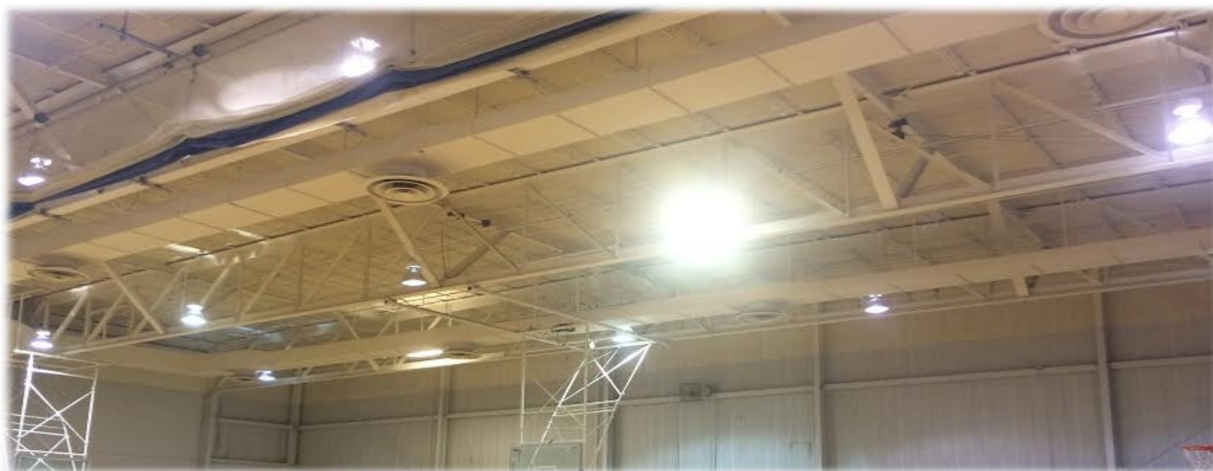
Figure 1: The current HID lights in Walzel Gym compared to the LED sample light installed this semester (in the middle). HID output is approximately 45 foot candles, LED is approximately 65 (LED model: Holophane Vantage).
